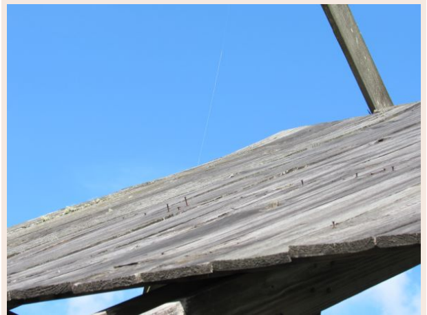
Example of repair/maintenance needed at the fishing pier: warped roof and loose roof nails.
