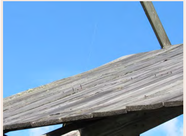
Example of repair/maintenance needed at the fishing pier: warped roof and loose roof nails.
